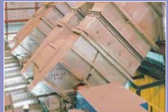
Fans on iron ore processing plant require a high degree of abrasion resistance
