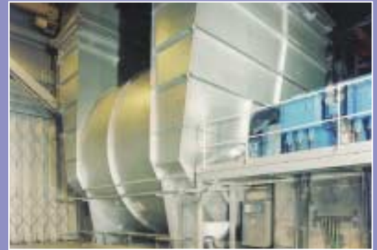
Fans on many power stations now operate for four years between outages
